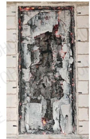
Fig. 6 Exposed Side after 60 Minutes of the Fire Test 1
