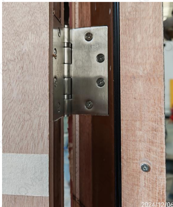
Photo 4 – Hinge and Intumescent Strip
