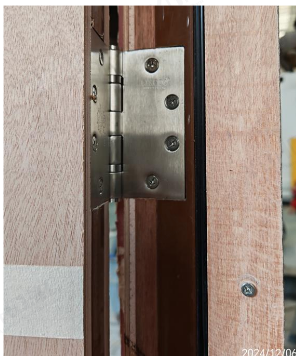
Photo 4 – Hinge and Intumescent Strip
