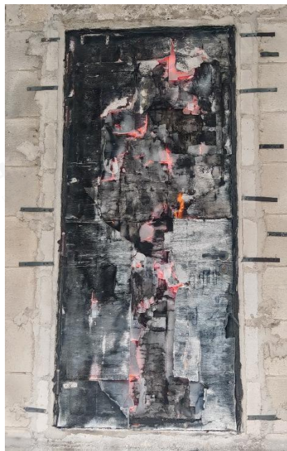
Fig. 12 Exposed Side after 60 Minutes of the Fire Test 2
