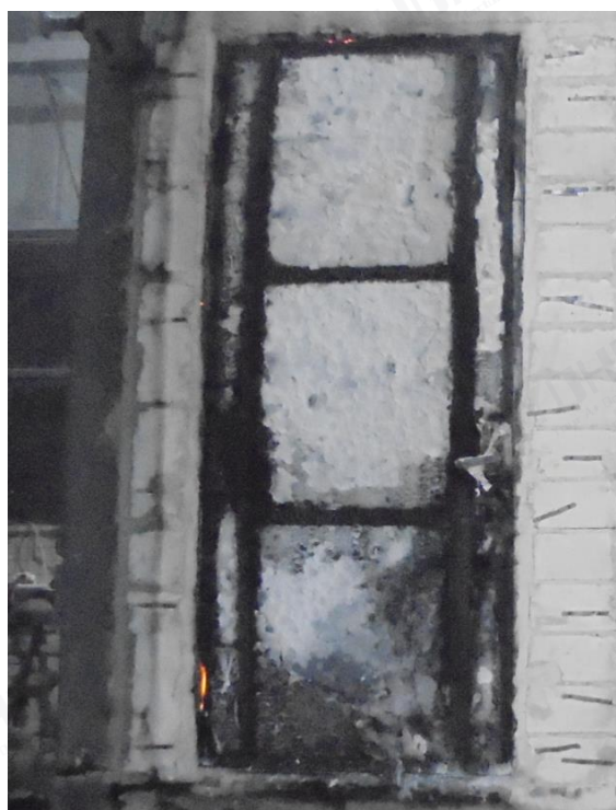
Photo No. 6 Exposed Side after 60 Minutes
