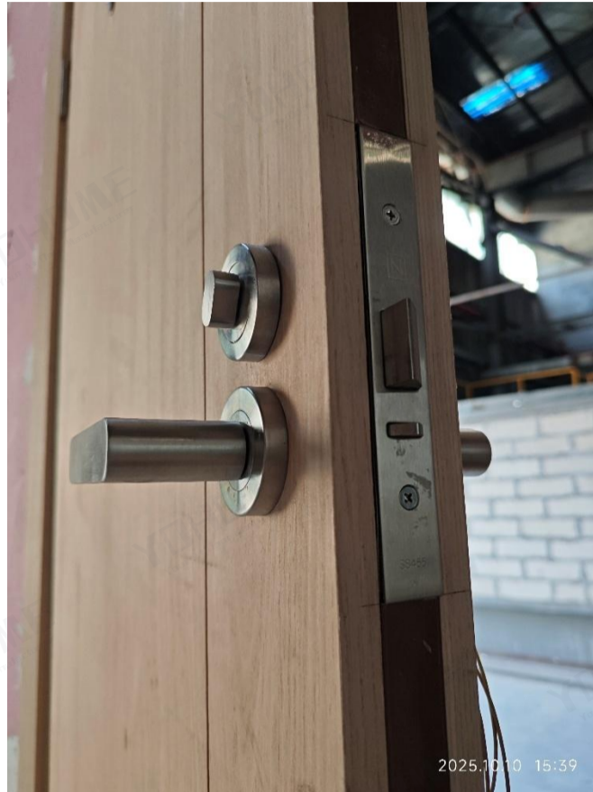
Photo 3 – Latching Mechanism and Intumescent Strip
